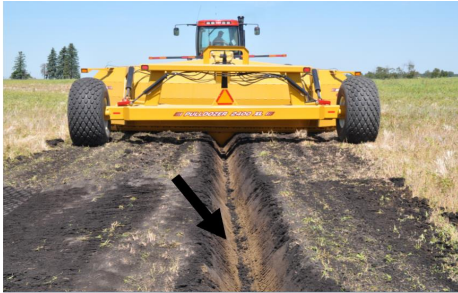
Figure 2.4 – Trench after the operation with no wind row ridges of dirt left
